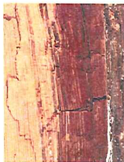
Figure 254. Advanced decay of Douglas-fir wood.
